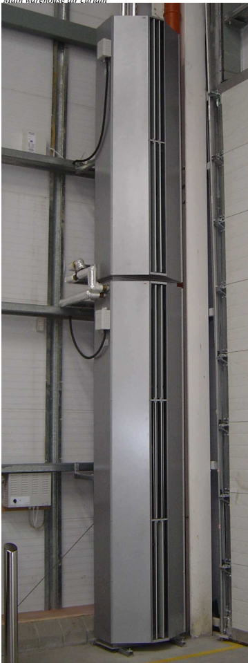
Main warehouse air curtain
