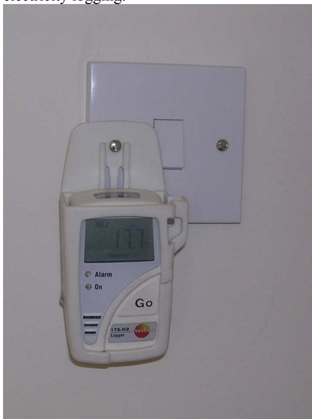
Temperature and relative humidity logger
